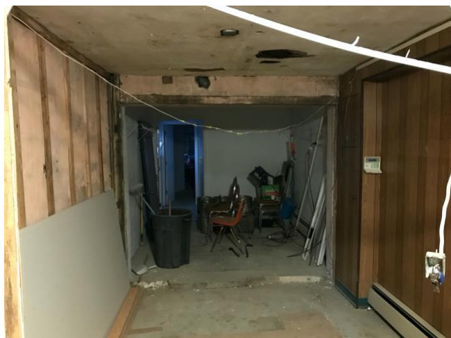
The coat closet is gone (new bathroom walls are in the far background)
